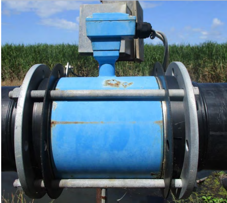
In-line Flow Meter
