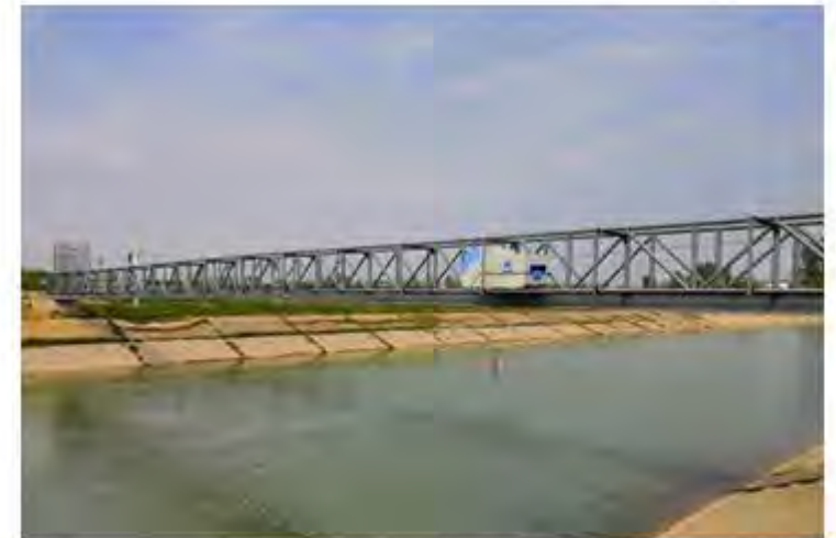
灌区渠首安装的流量计量设备 Flow-measuring equipment installed at the headwork of an irrigation scheme
