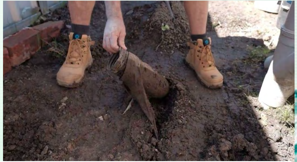
Geotech fabric also becomes blocked
