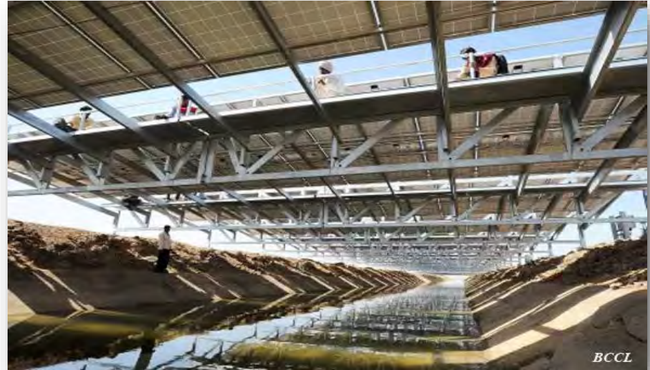
India's first 1MW canal-top solar power plant at Chandrasan village near Mehsana, 45 kms from Ahmedabad on World Earth Day, April 22, 2012. (BCCL)
