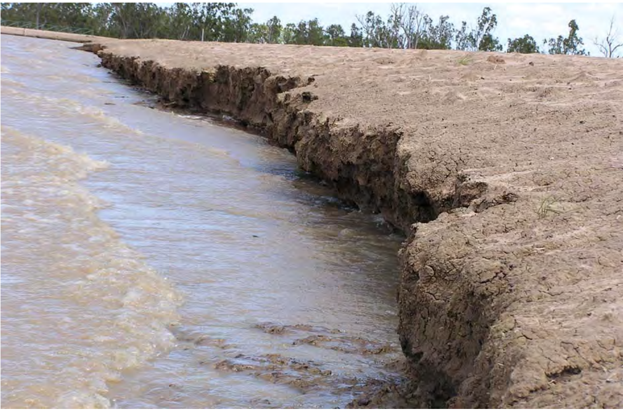
Figure 5.4 Wave erosion on the inside batter
