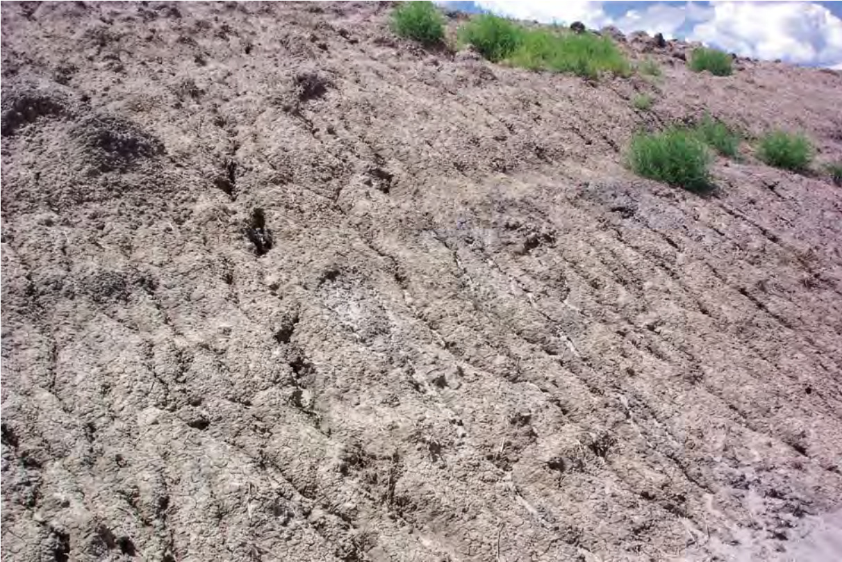
Figure 5.3 Rills as a result of erosion on the outside batter
