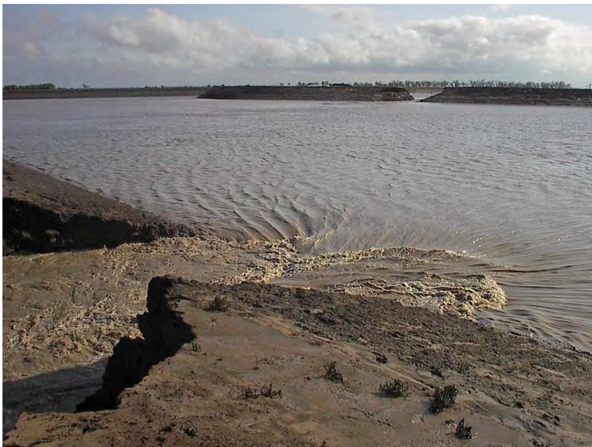
Figure 2.1 An irrigator's worst nightmare – a breached storage embankment
