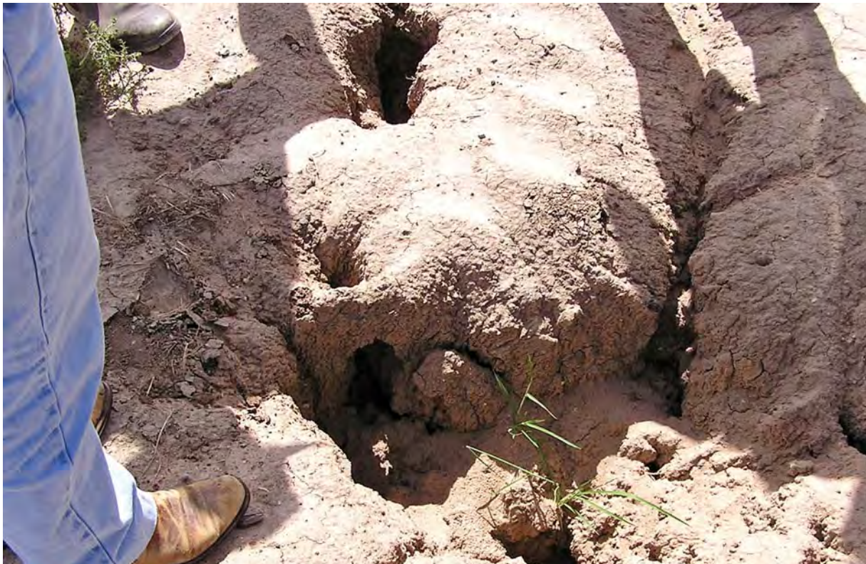
Figure 5.2 Cracking, erosion and tunnelling of embankment crest
