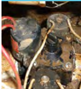
Poorly Maintained Solenoid Valve
