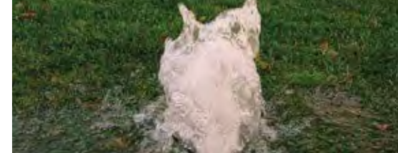
Broken Irrigation Pipe
